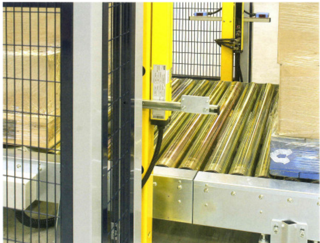
Automatic light curtain protection preventing entry to the danger zone but allowing exit of a full pallet.
