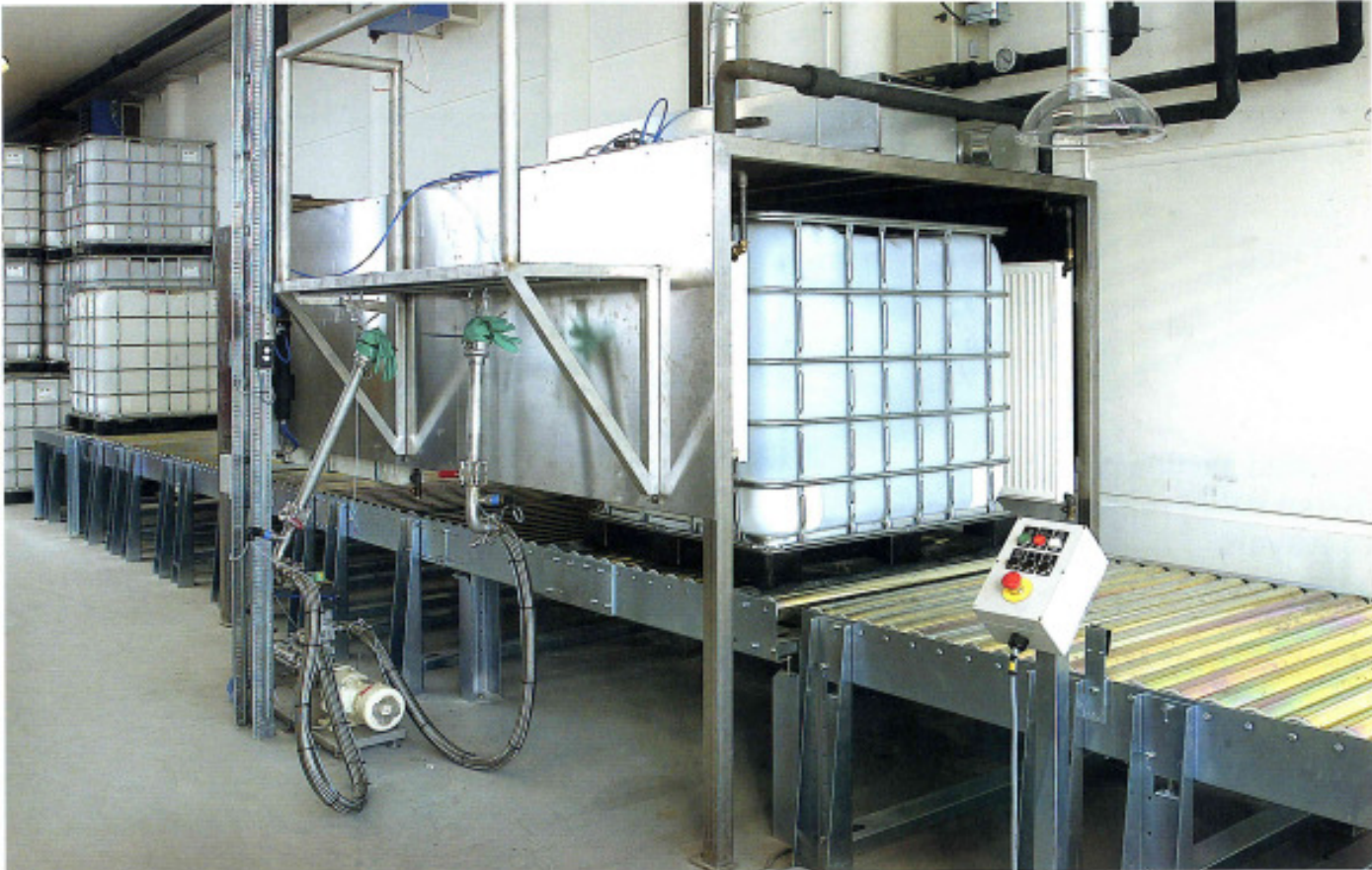
Pallet conveyor system for handling of pallet containers with liquids at Coloplast in Denmark.
