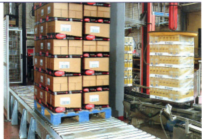
Driven pallet conveyor system at Dansk Kaffe Kompagni in Denmark.
