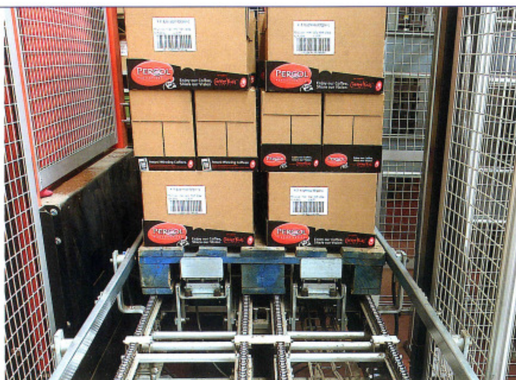
Simplex chain conveyor system at Dansk Kaffe Kompagni, Denmark.
