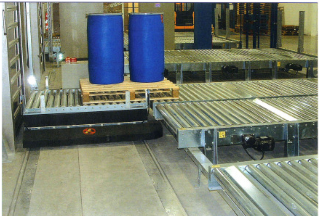
Transfer trolley installed in a pallet roller conveyor system supplied to Organon, Ireland.
